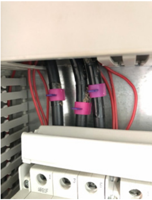
3-phase intake supply into distribution board
